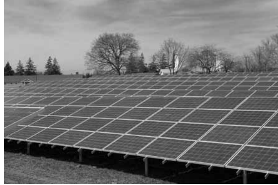
Large solar-panel installation on the Livingston Campus of Rutgers University in Piscataway, New Jersey.
